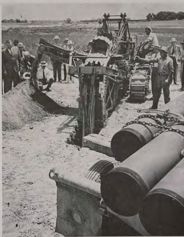
Big ditching machine is here shown excavating for the Texas section of the Longview-Salem 550-mile, 24-inch pipe line, now under construction. Standing at end of conveyor is County Judge Merritt H. Gibson and bending over beside him is Carl L. Estes, recently commissioned a lieutenant commander in the U.S. Navy. Other Longview civic leaders are seen in the background.
